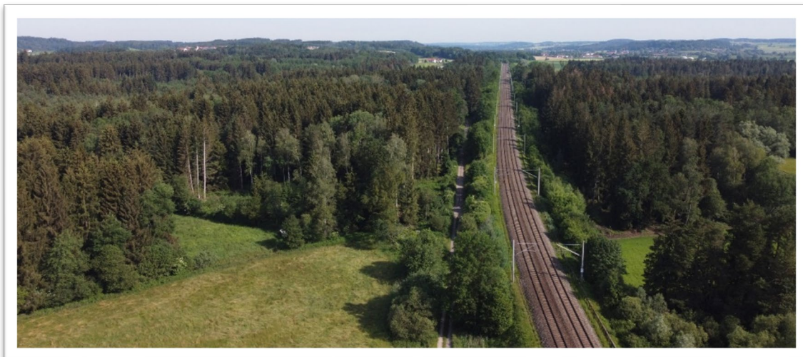
Caption: In the Grafing-Ostermünchen section, a new line is being built as the northern approach to the Brenner Base Tunnel. Source: DB Netz AG
