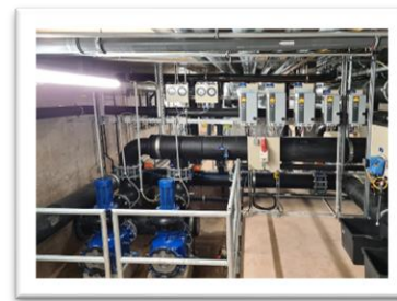
Bath water technology, circulation pumps
