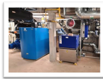
Boiler and combined heat and power unit
